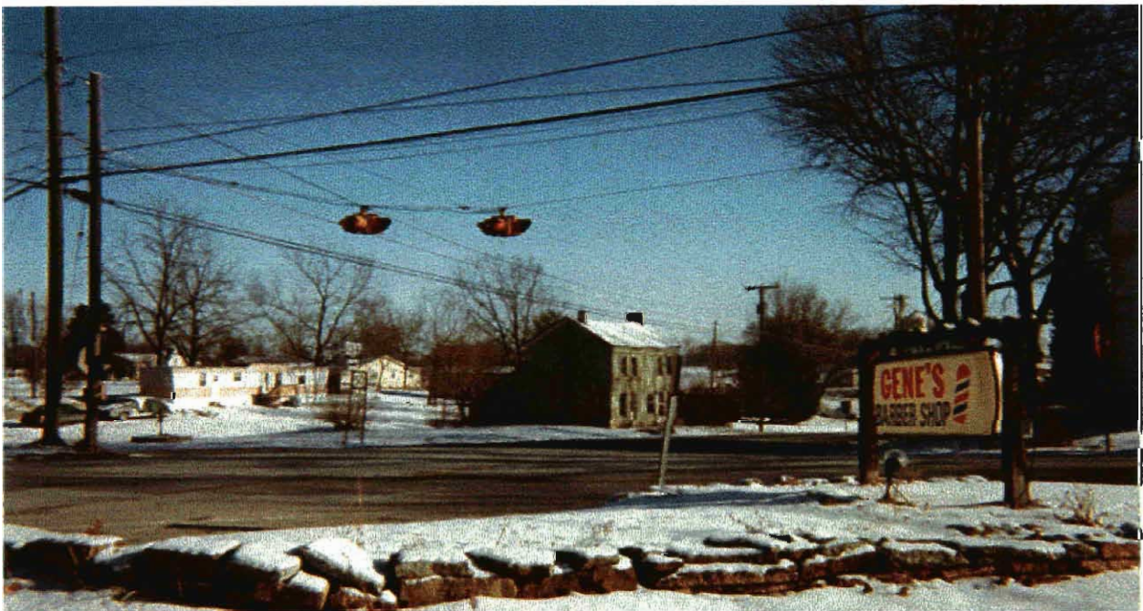
INTERSECTION CONTROL BEACON (WEST INTERSECTION)
